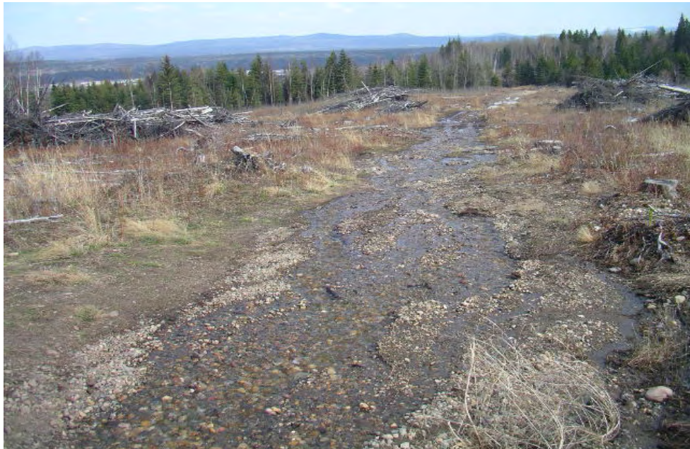
Photo 6. Erosion caused by logging practices East of Tyner Boulevard within Stream B.
