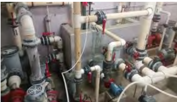
Mechanical room piping
