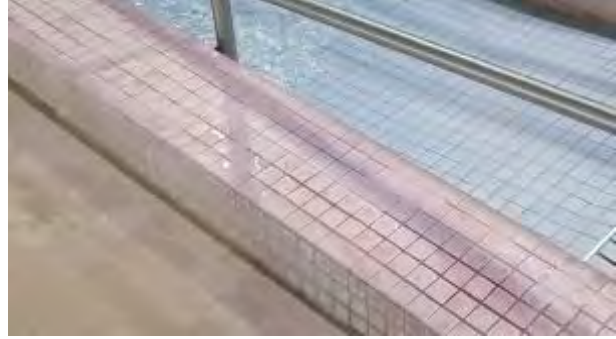
Stained tile at spa
