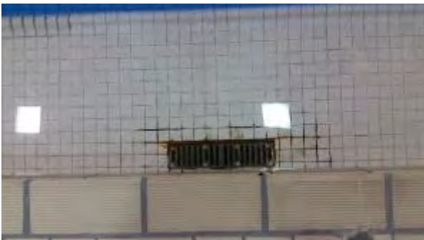
Corroding gutter dropout grate
