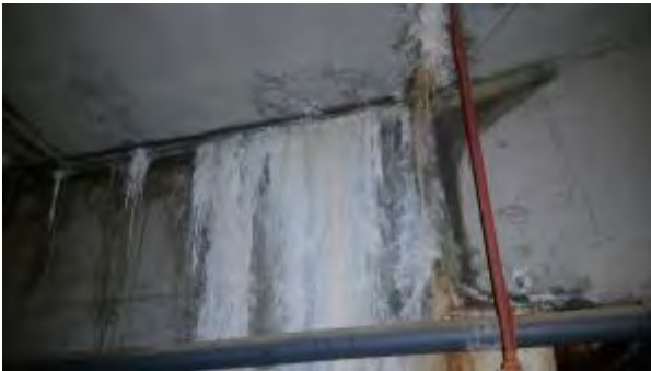
Leaks in pool shell
