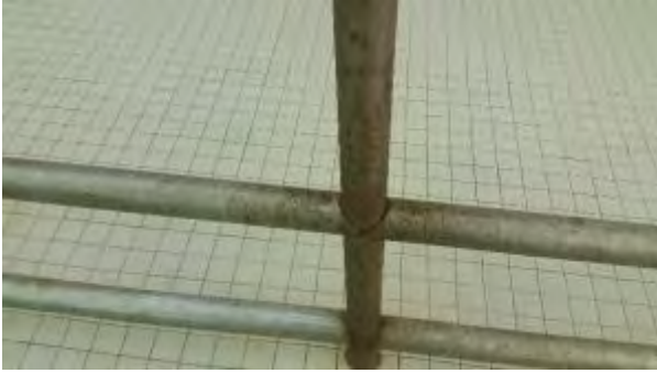
Corroding rail goods
