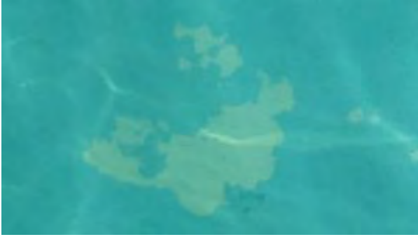
Chipped plaster finish in recreation pool
