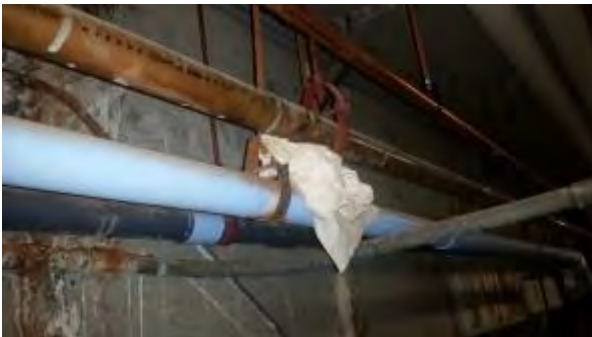
Mechanical room piping
