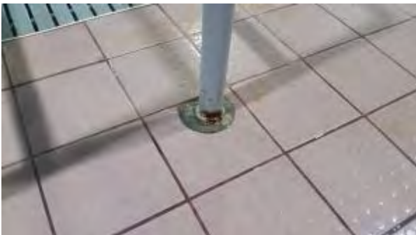
Corroding rail goods
