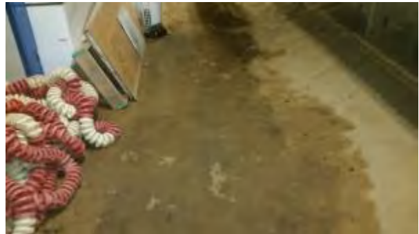
Wet mechanical room floor
