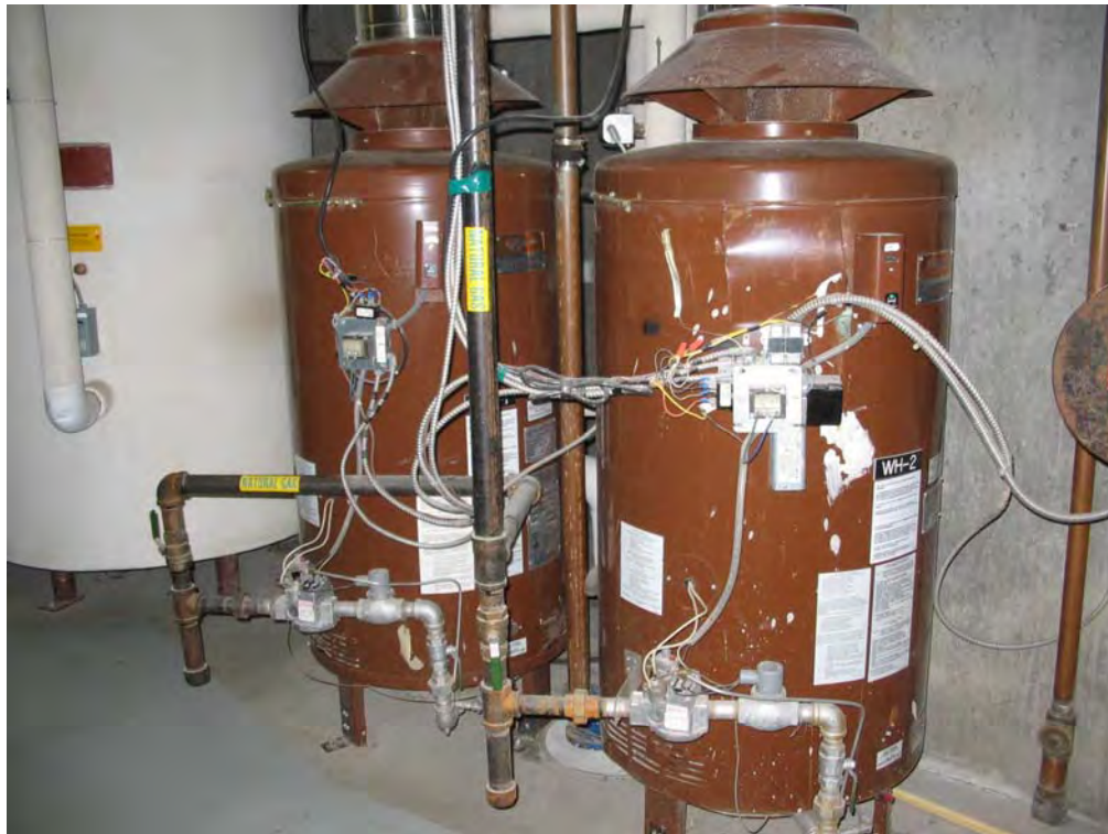
Figure 20: Two out of three of the atmospheric hot water heaters
