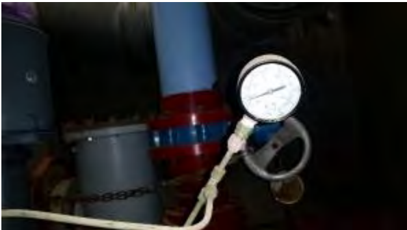
Broken pressure gauge
