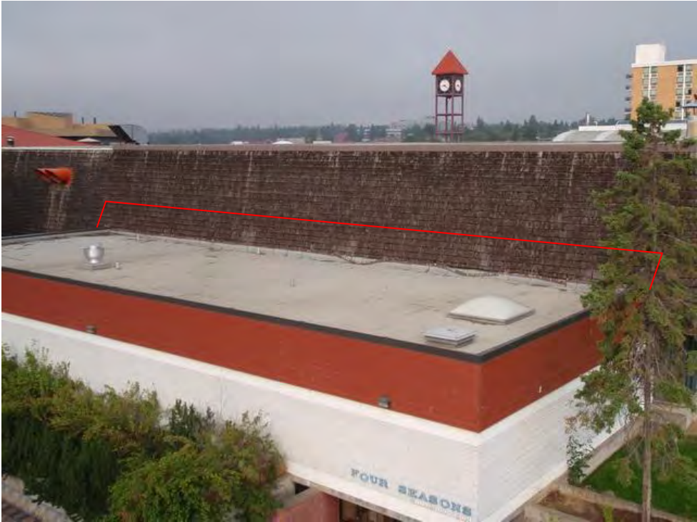
Photo 5: East Mansard roof above change areas. Red line indicates minimum area of temporary remedial repair.
