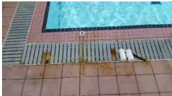
Stained gutter grating on lap pool
