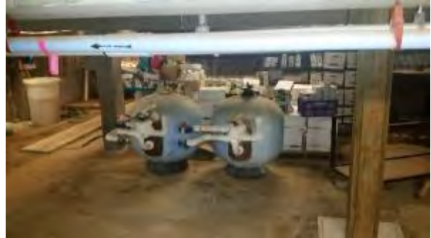
Abandoned pool equipment
