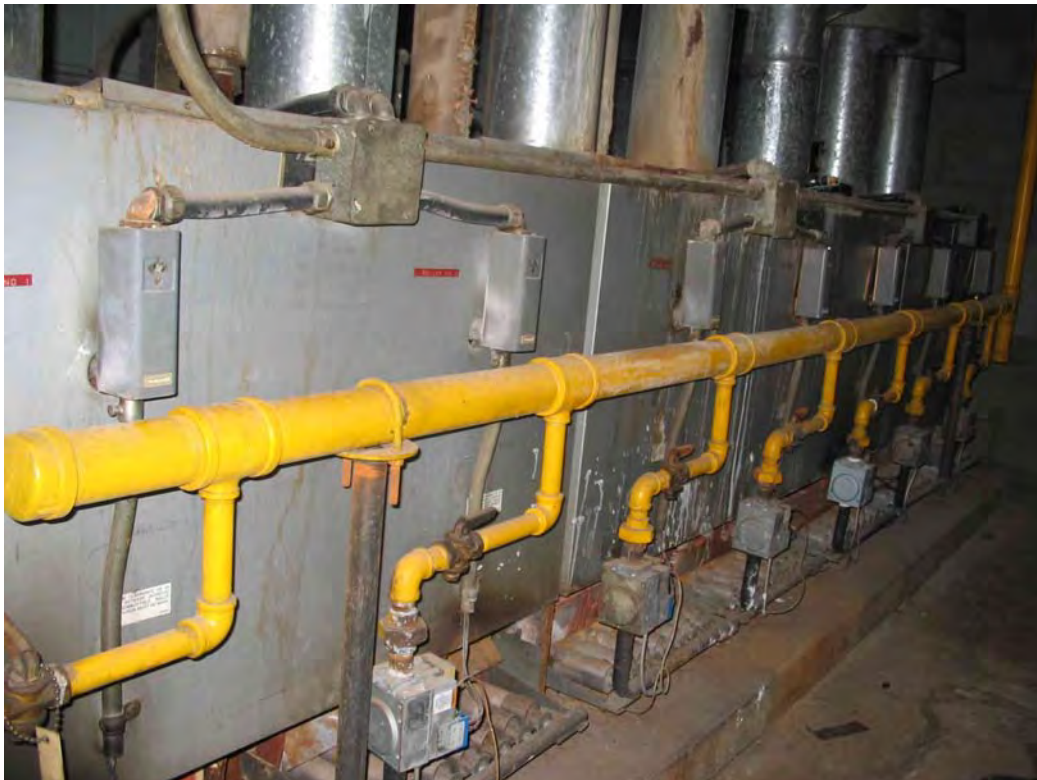
Figure 6: Inefficient atmospheric boilers – Four Seasons Pool
