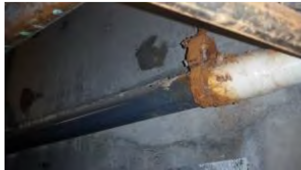
Corroding pipe hanger
