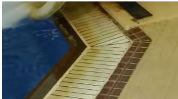
Stained gutter grating
