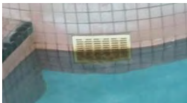
Stained skimmer inlet grating in recreation pool
