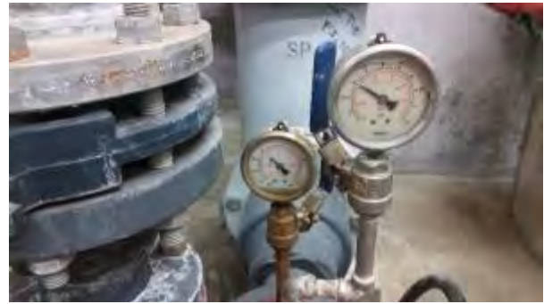
Vacuum and pressure gauges
