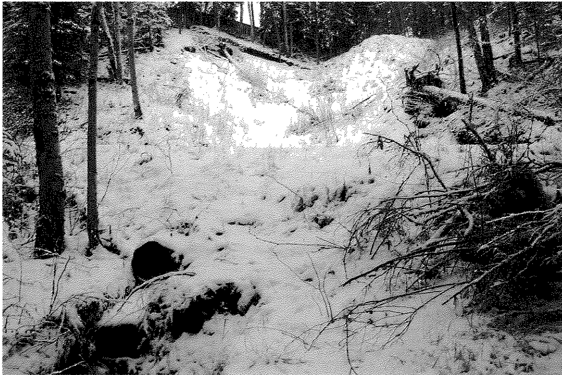
Photograph 4: View of soil erosion of slope above a storm sewer outfall below Essex Crescent.
