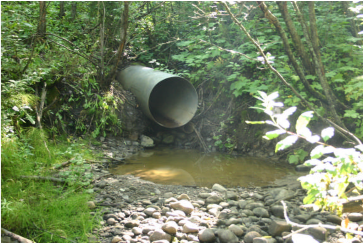
Plate 1. Date: Aug. 4, 2004. Comments: 0.4 m hanging culvert barrier on Zogas Creek at the Highway 97 crossing.
