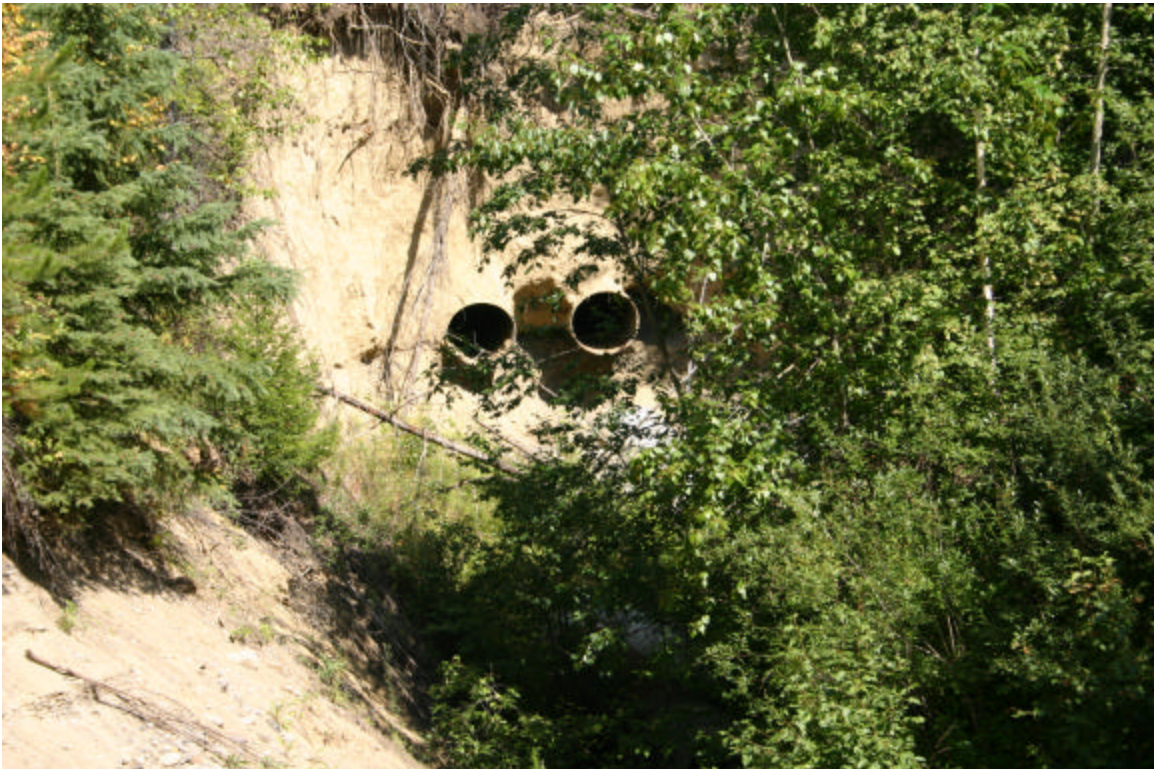
Plate 2. Date: Aug. 4, 2008. Comments: Twin 1200 mm hanging culverts (1.6 m high) on Unnamed Creek 2 at old road crossing ~220 m upstream of the Fraser River.
