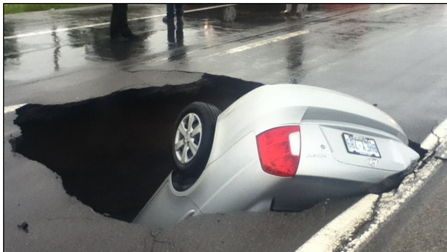
Figure 5: 2012 Sinkhole In Ottawa
