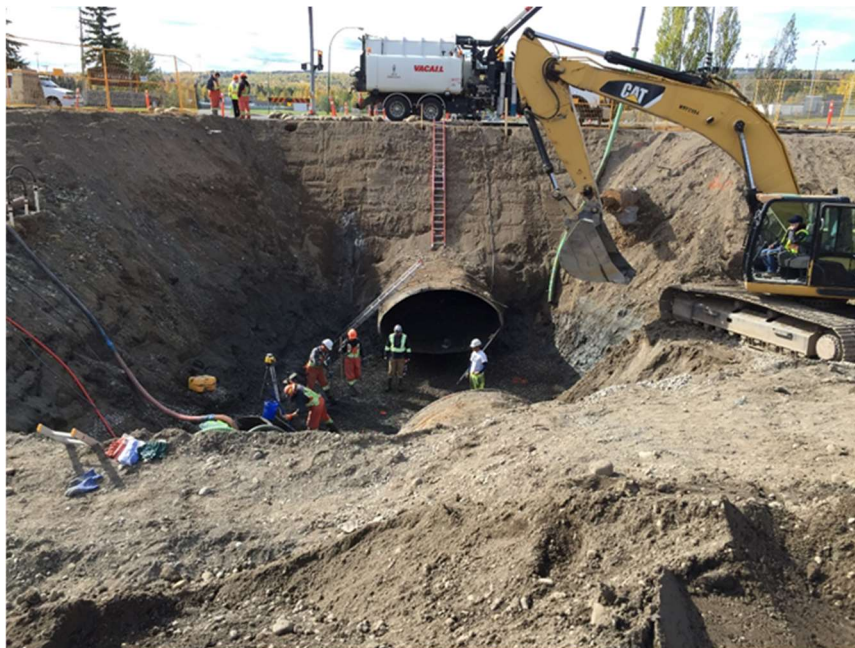
Figure 5: Winnipeg St. Sinkhole (2018) - $1.7M
