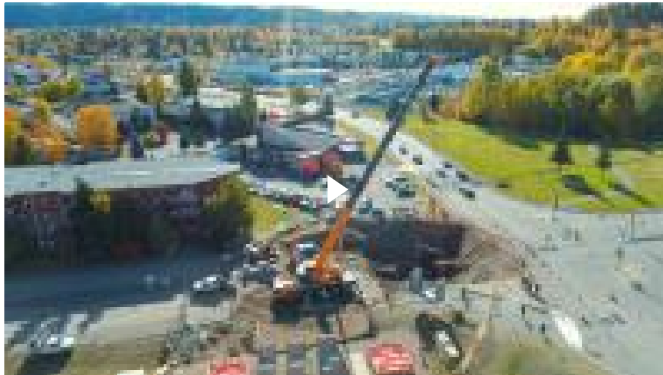
Winnipeg St. Sinkhole
