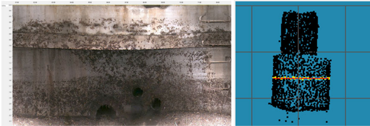
Figure 22 Manhole Panoramic Inspection Results
