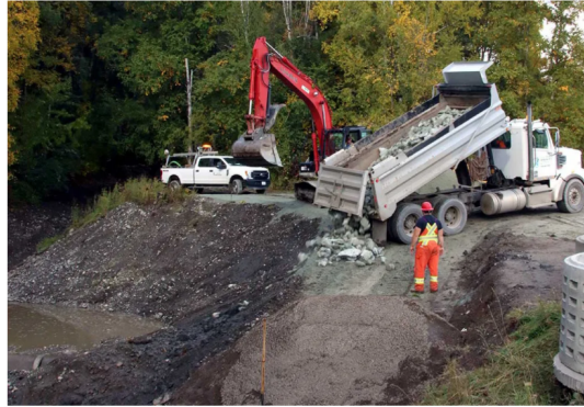
City crews conduct an operation to remediate a stormwater pond near the bottom of Shane Creek in Ginter's Meadow – an example of work the city does to maintain its stormwater infrastructure. City of Prince George photo
