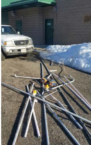
PW 601 Wilson Park East Well Fluoride Injection System Equipment Removed
