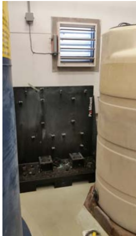
PW 660 Fishtrap Well Fluoride Injection System Equipment Removed
